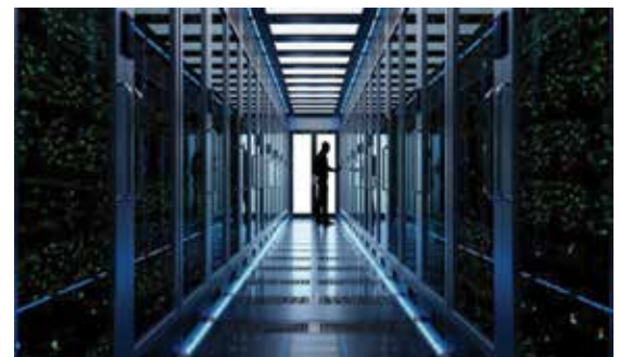
Data Centre Infrastructure & Monitoring Solution
