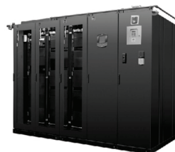
Smart Data Center
